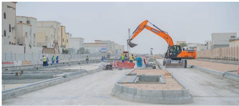
The project relies on local materials and manufacturers, with the local component accounting for 85% of the total materials used.
