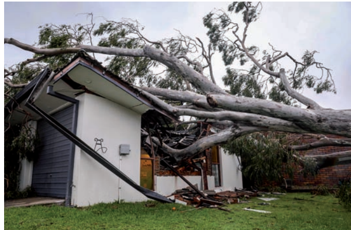
A damaged home is pictured after a tree uprooted by strong winds crashed into the structure in the suburb of Elanora as Cyclone Alfred passed near the Gold Coast yesterday. (AFP)
