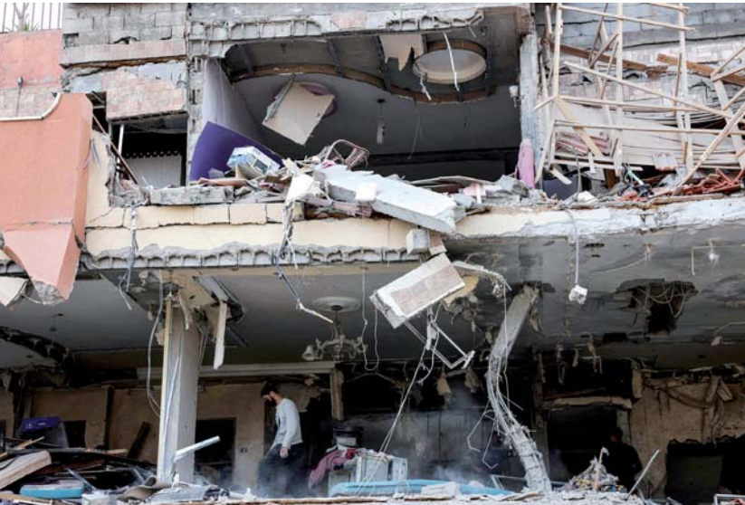
A damaged building is pictured after an Israeli air strike in Gaza City yesterday. (AFP)
